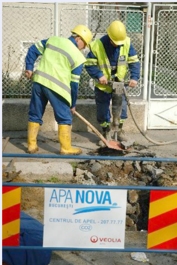
Working on a water connection in the Bucharest. (Photo courtesy of Apa Nova)
